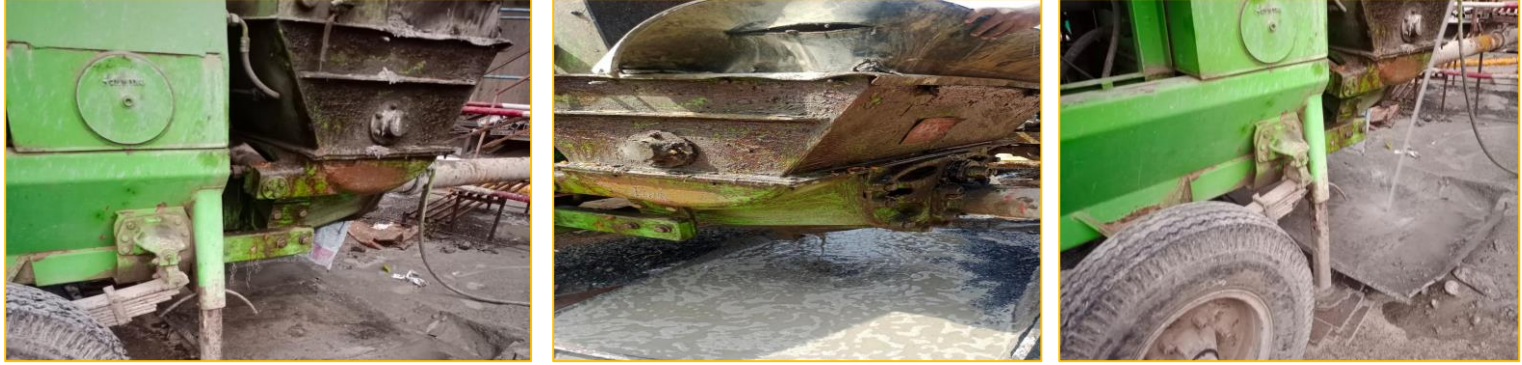
Deep Tray Provision is being followed at site for concrete pump wash to prevent soil contamination.
