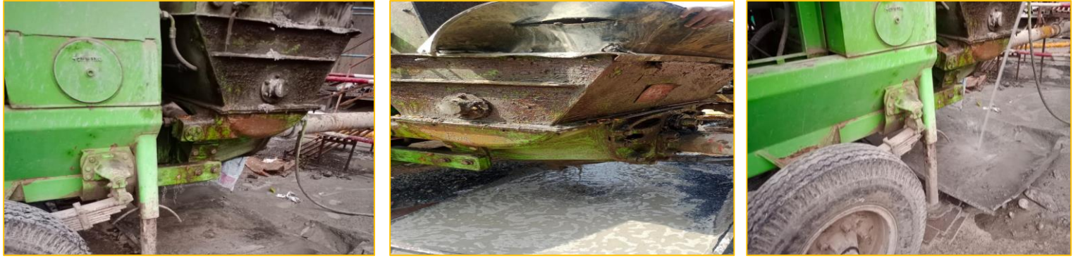
Deep Tray Provision is being followed at site for concrete pump wash to prevent soil contamination.
