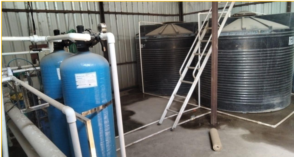
RO Plant installed in Workmen Camp for drinking water.
